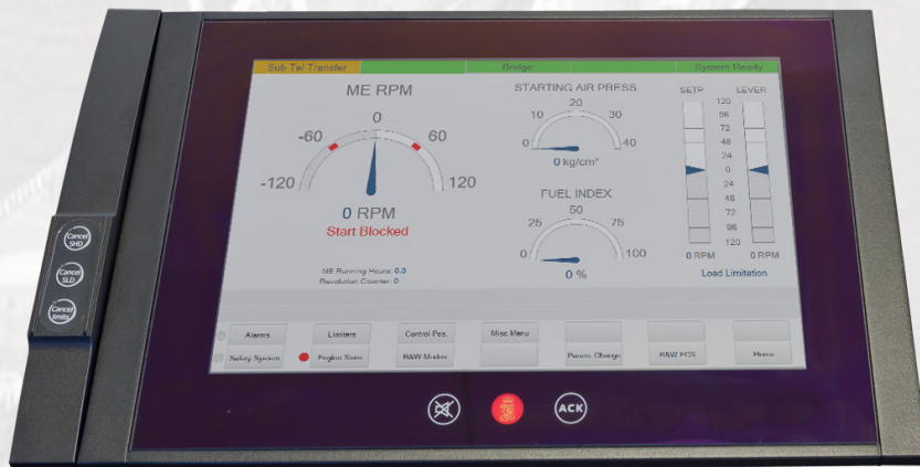
The AutoChief® Control Panel
