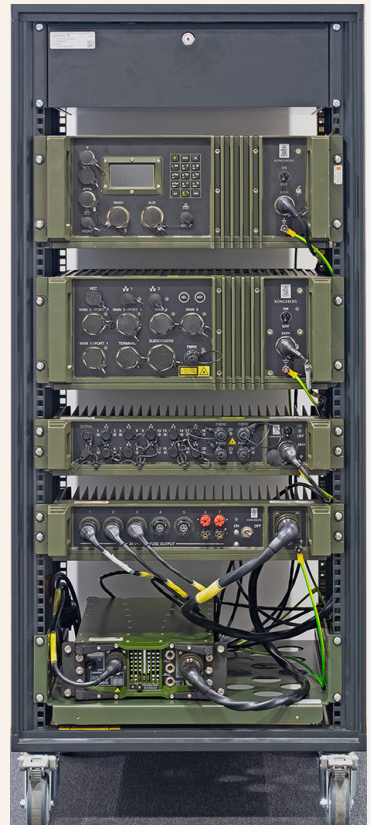
K-TaCS communication rack
