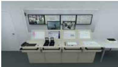
Engine control room
